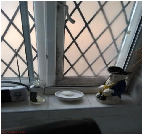
Condition of bathroom window at initial inspection (below)
