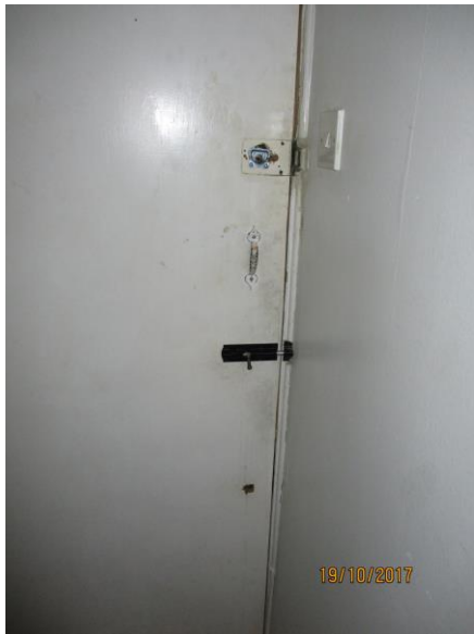
Lock missing to flat entrance door
