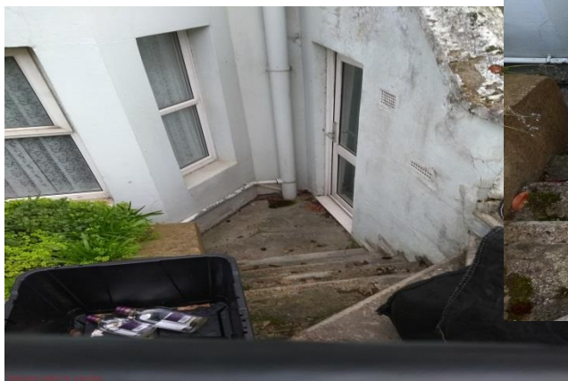
Condition at Initial Inspection
