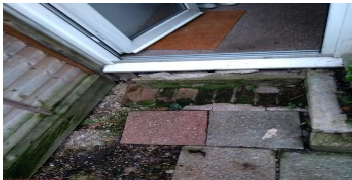
Condition at initial inspection
